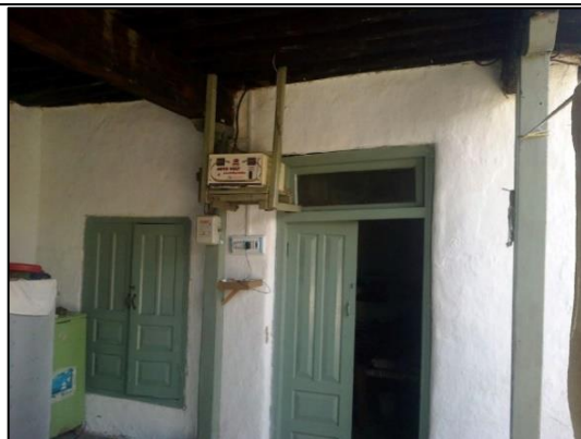
Figure 15. Highlighting mud/cladding on the interior
