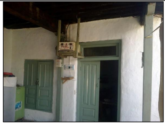
Figure 15. Highlighting mud/cladding on the interior
