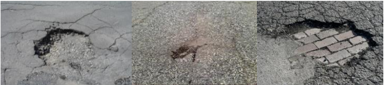
Figure 1. Road image(s) with Pothole [1]
