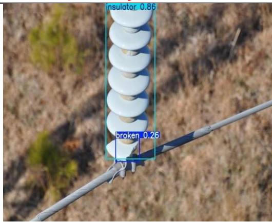
Figure 4. Detection of a Broken insulator using YOLOv8m with accurate localization.
