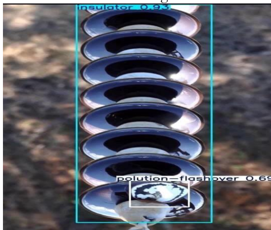
Figure 5. Detection of a Pollution Flashover defect using YOLOv8m.
