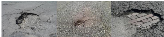
Figure 1. Road image(s) with Pothole [1]
